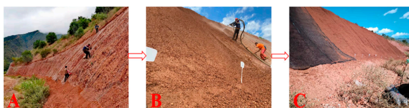
Figure 2. The process diagram of the soil spray-sowing technique, including the hanging net (A), soil spray-sowing (B), experiment treatments, and labeling (C).
